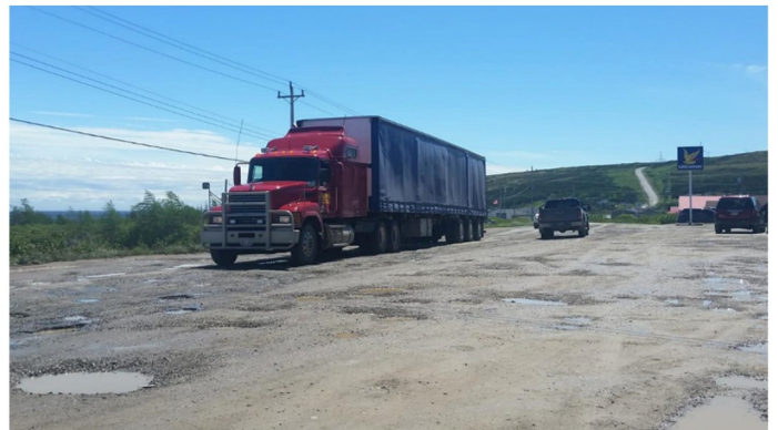
Figure 3: Potholes on highway 510 in Forteau NL, July 2017.
